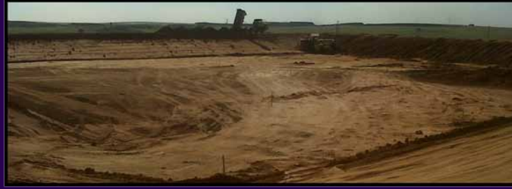
SUDOR COAL: POLLUTION CONTROL DAM
